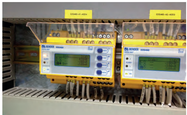
MES-Engineering with solutions from Bender in PVD rig project
