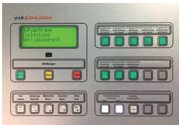
In 2004: TM1000 with monitoring of eight IT systems and lighting group controllers
